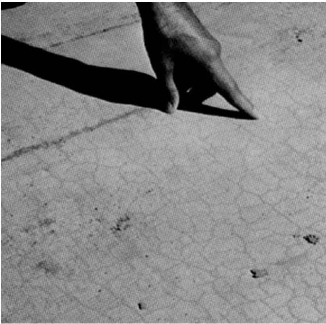
Figure 4. Crazing is a network of fine surface cracks. (4099)
