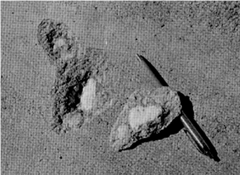
Figure 8. A popout is a small fragment of concrete surface that has broken away due to internal pressure, leaving a shallow, typically conical, depression. (0113)
