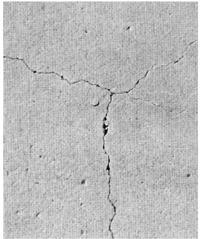
Figure 3. Drying-shrinkage cracks like these often result from improper joint spacing. (A5271)
