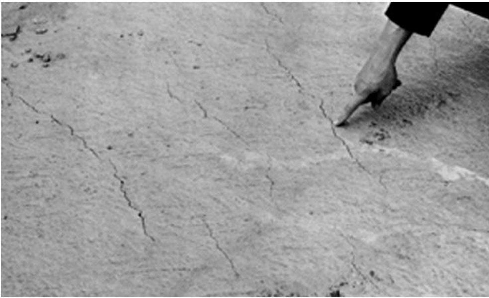
Figure 2. Plastic-shrinkage cracks caused by rapid loss of mix water while the concrete is still plastic. (1311)
