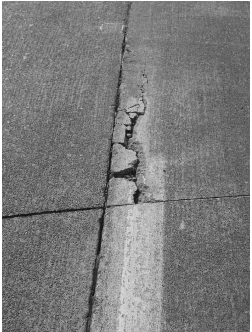
Figure 11. A typical location for a spall is along a joint, usually the result of the joint functioning improperly. (67216)
